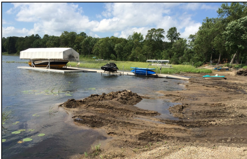
Example of work conducted without a permit and in violation with District Rules, Shoreland Ordinance Rules, and MN DNR Waters regulations.
