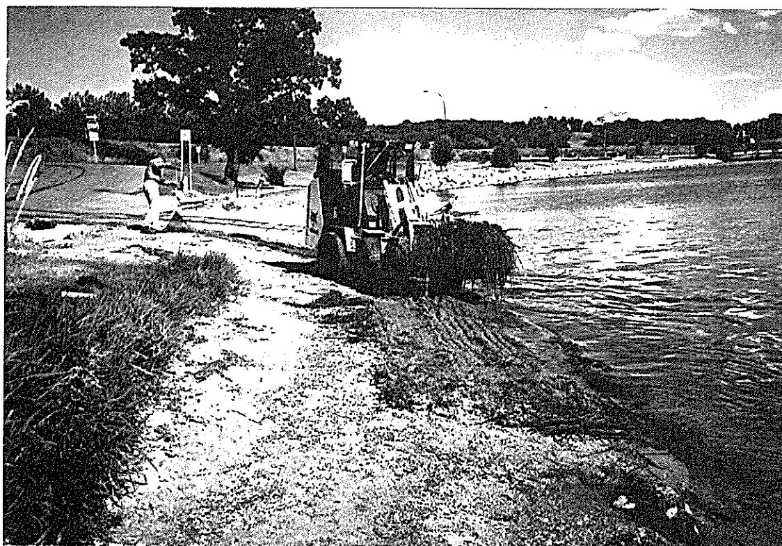
Figure 10. (Top) Plants are transferred to a dump truck. (Bottom) When pick up is finished, the shoreline is clean.
