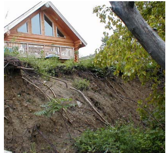
This is an example of eroded bluff in Meeker County.
