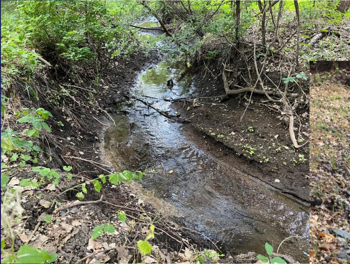
Before : Erosion & Failing Banks
